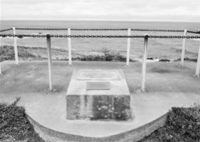
The Honda Point Memorial site is currently off-limits. Due to erosion from the Pacific surf, the surrounding cliffs are severely undermined
